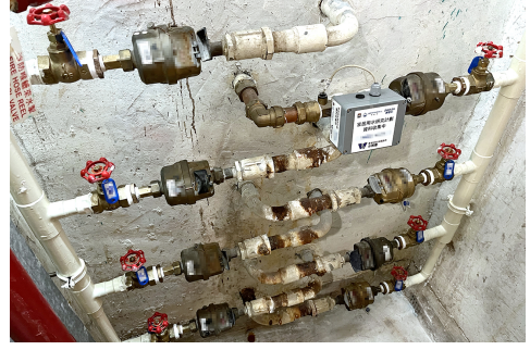
(b) Confined environment of a typical meter room
