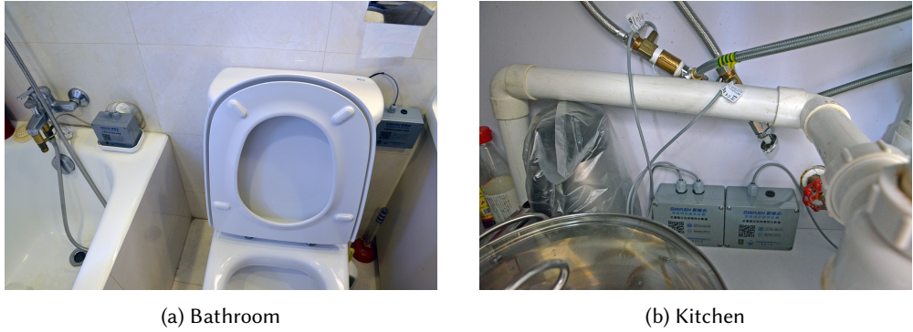
Fig. 8. Example Tap Sensor and Flush Logger installations inside an apartment
